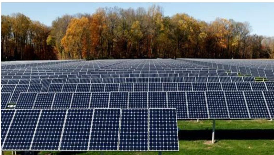
Figure 1. The solar farm's geometry shows a repeating range that produces periodic flow [2].
