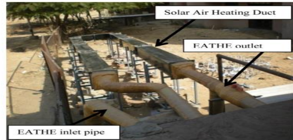
Figure 1. Experimental set-up of EATHE coupled with solar air heating duct.
