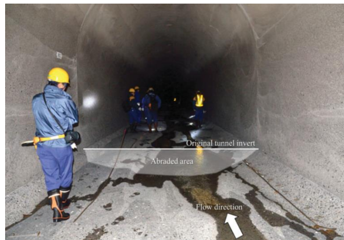
Fig. 1 Abrasion of the concrete invert the Asahi SBT [8]
