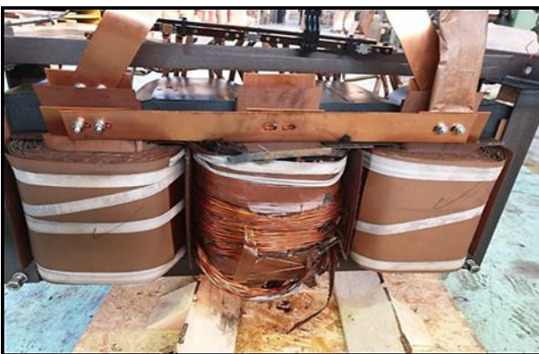
Figure 2. Destroyed windings after short circuit current
