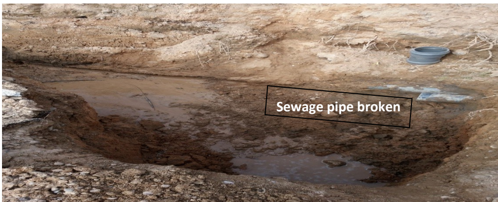
Plate 3 (B) sewage pipe broken
