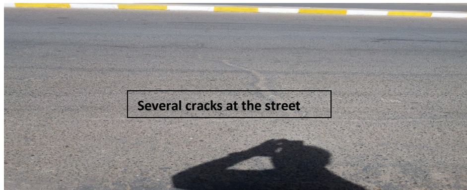
Plate 2(A) Several cracks at street near girls education college
