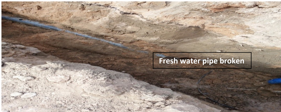
Plate 3 (A) Fresh water pipe broken
