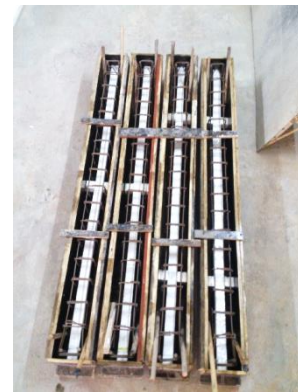
Fig (7): Mobilizing of BLTO Prototypes before Casting by Fastening Reinforcement Cages and Styropor with Temporary Covers Inside the Plywood Molds.
