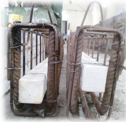
Fig (6): Reinforcing Steel Cages of 2-Referential Prototypes to Choose the Optimum Zone of Hollow Core Section.
