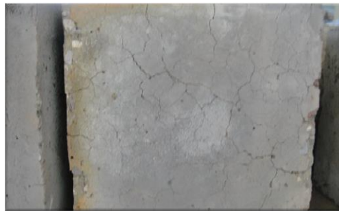
Figure 4. The surface of the cub with GL51 after 1 hr fire
