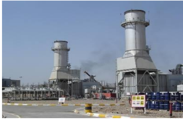
Figure 1. Power station of south of Baghdad.
