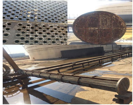
Figure 2. Fouling of heat exchangers (AL-Daura Refinery).
