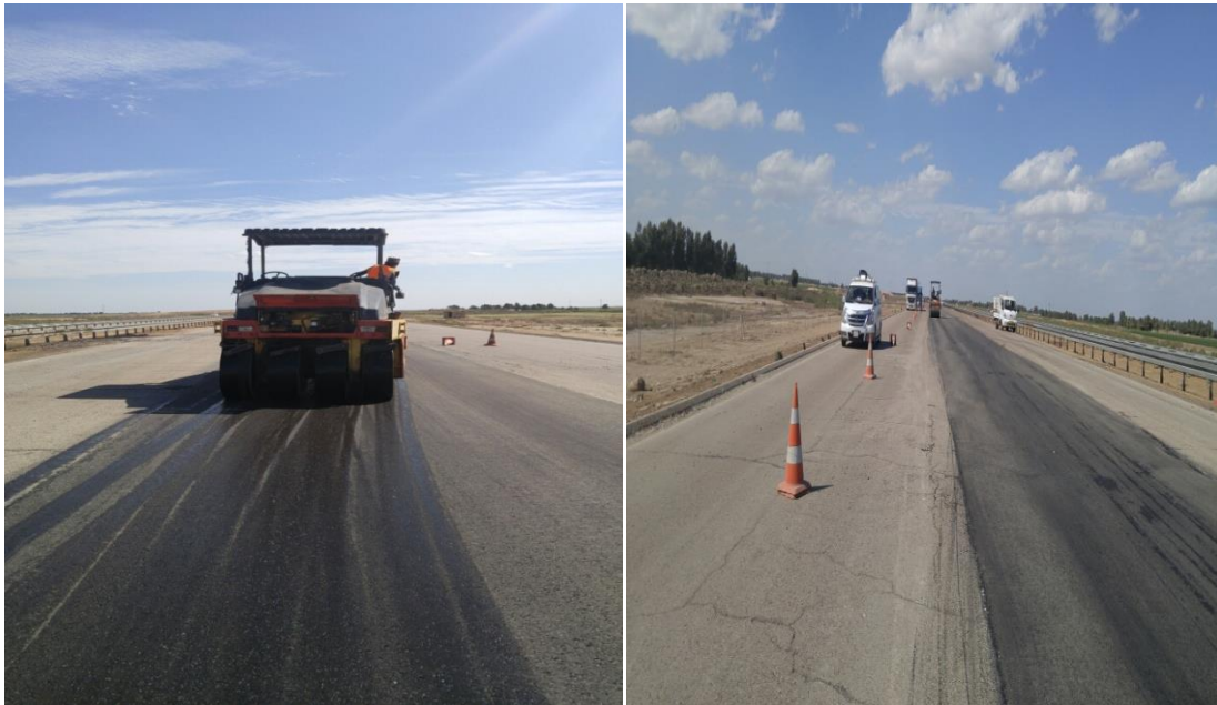
Figure 7. Using of modified hot mixture asphalt in the paving of highway surface course
