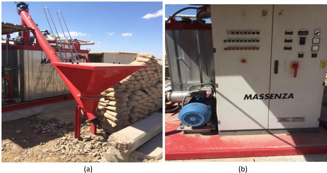
Figure 2. Mixing machine of SBS with asphalt within hot mixture asphalt plant in site of project
