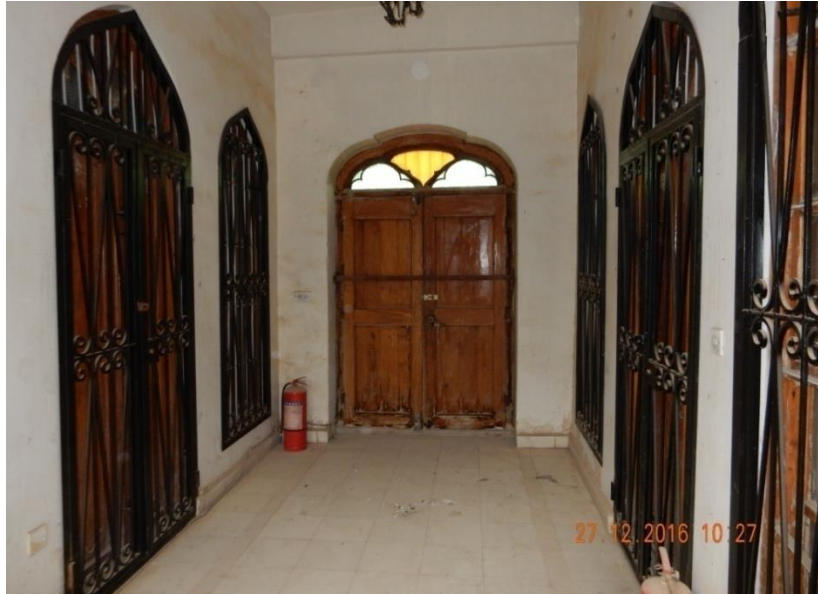
Figure 12. The problematic use of Portland cement in repairs
