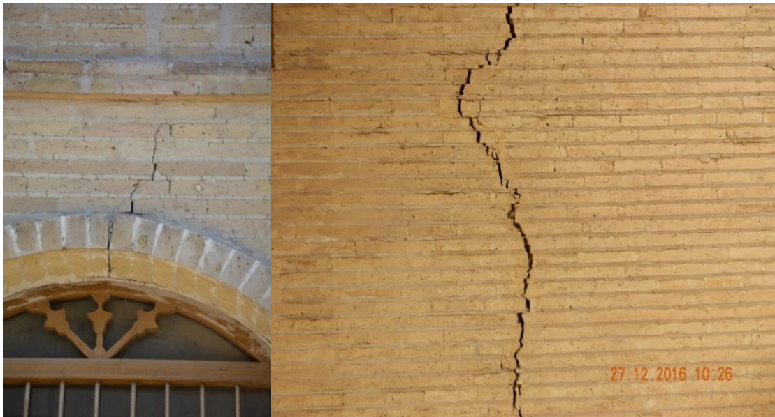
Figure 11. Cracks in two historical houses in Baghdad.
