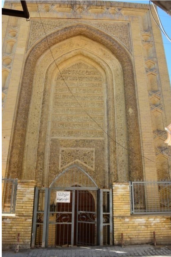
Figure 8. Example on bad conservation (new bricks do not match the old in color and texture)
