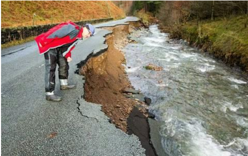
Fig.(1): Failure of hydrological design.
