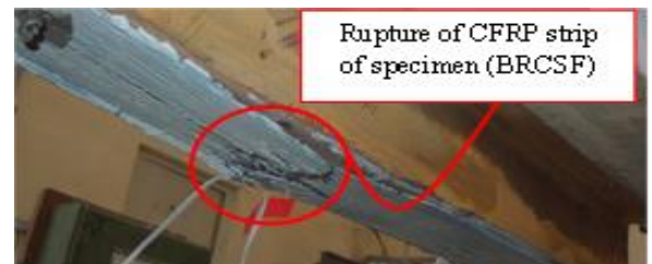
Figure 18. Mode of failure of beam BRCSF
