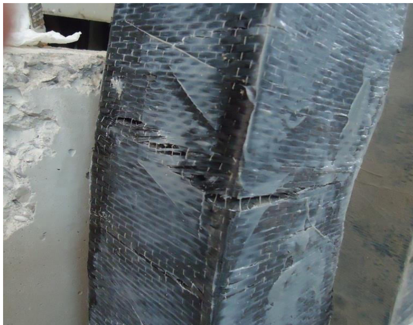
Figure (17) Rupture of CFRP Sheet at Failure
