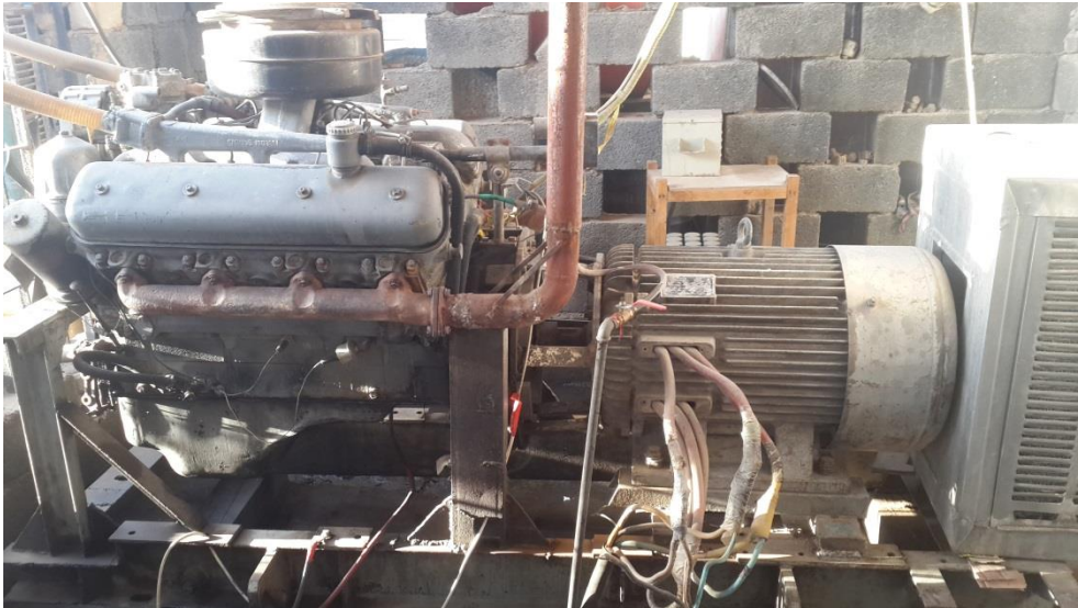
Fig.2 Show the connection of the engine and the induction generator by coplen
