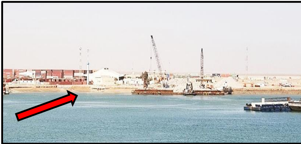
Figure 15. Construction of a 300 m long side wall to block the movement of waves and prevent sedimentation within the channel. Location: 30°03'50.5"N, 47°55'42.2"E, Photo date: 11/19/2021.
