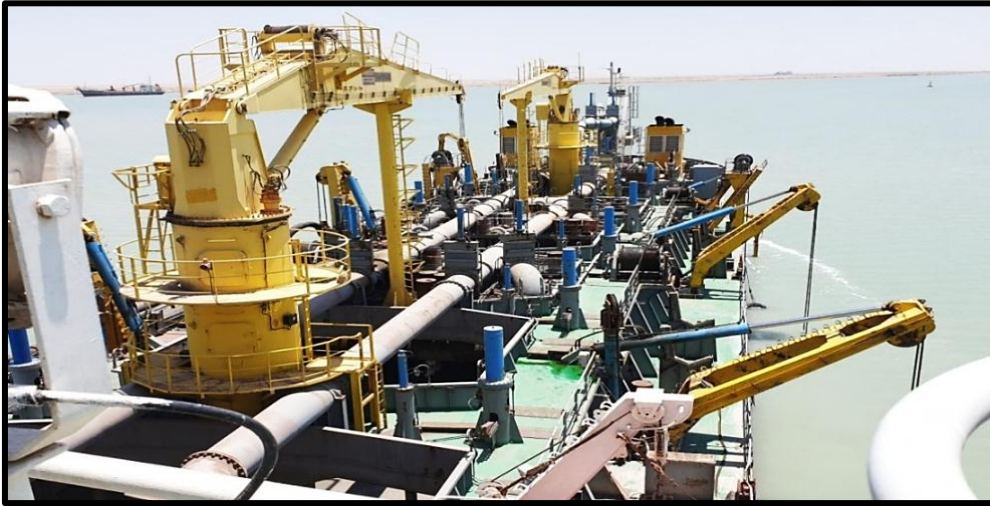
Figure 17. The process of dredging within the channel with the pelvic dredging rig. Location: 30°02'53.7"N 47°56'31.1"E, Photo date: 6/1/2022.
