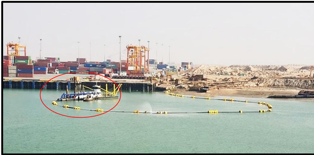
Figure 14. The shallow dredger barge is deepening the channel. Location: 30°03'28.4"N 47°56'08.0"E, Photo date: 9/1/2022.
