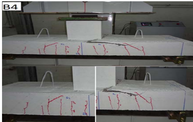
Figure (10) Crack pattern for (B4)
