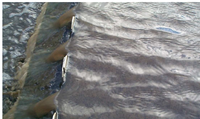
Figure 3. Overloaded clarifier operations
