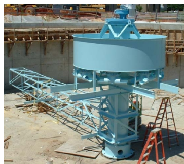
b) Picture of Modified center inlet structure (EDI)
