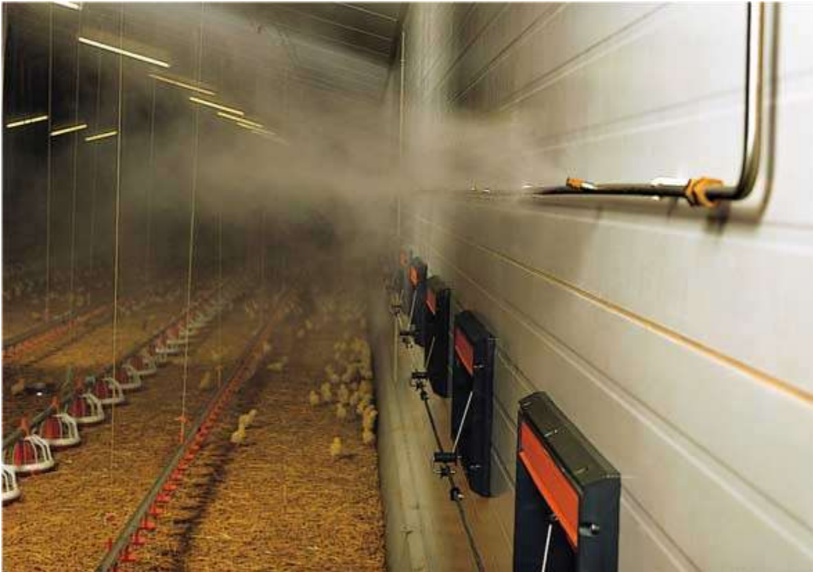
shows the use of water spray to reduce heat stress in poultry houses )6( .Picture No
