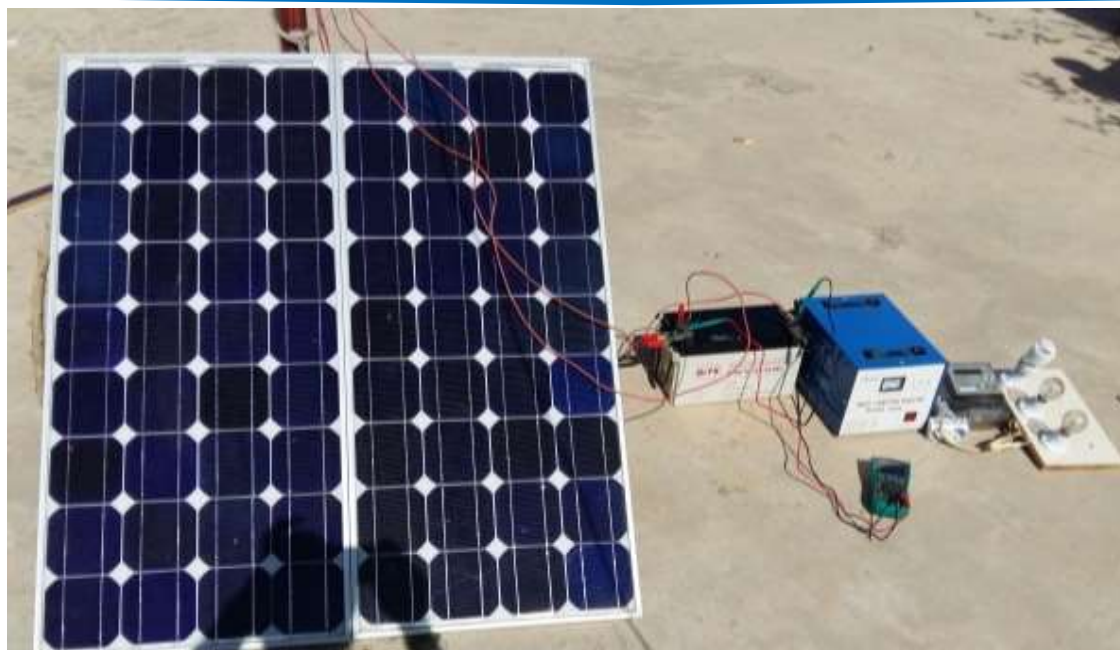
Figure 5 Energy generation by two solar panels of 80
