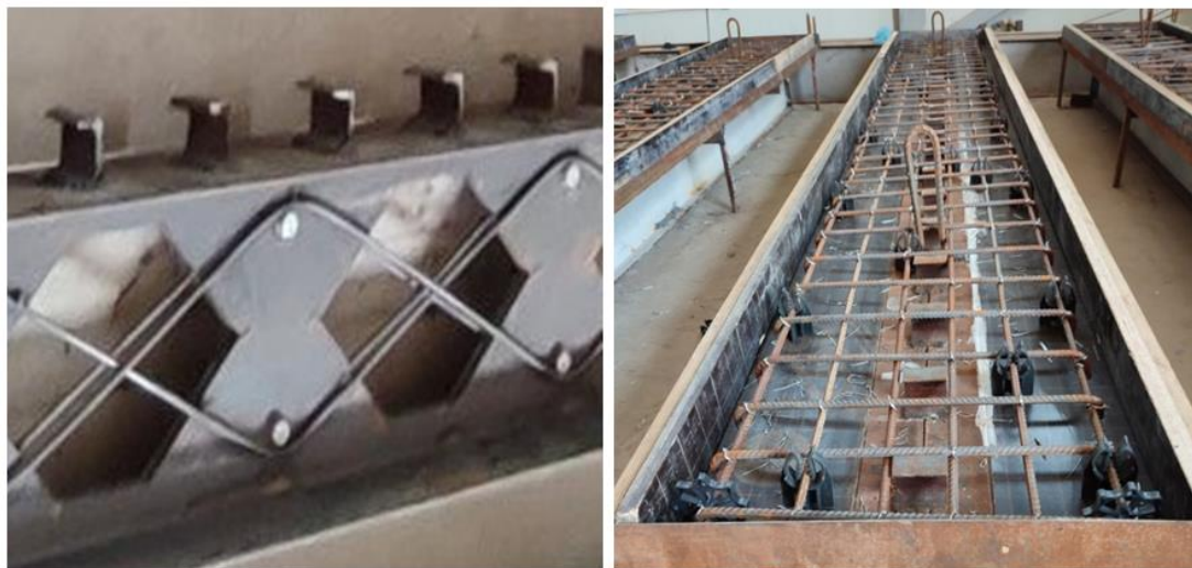
Fig. 8 The Steel Materials: A. Shear Connectors, Lacing, and Bolts, B. Deck Slab Reinforcement.
