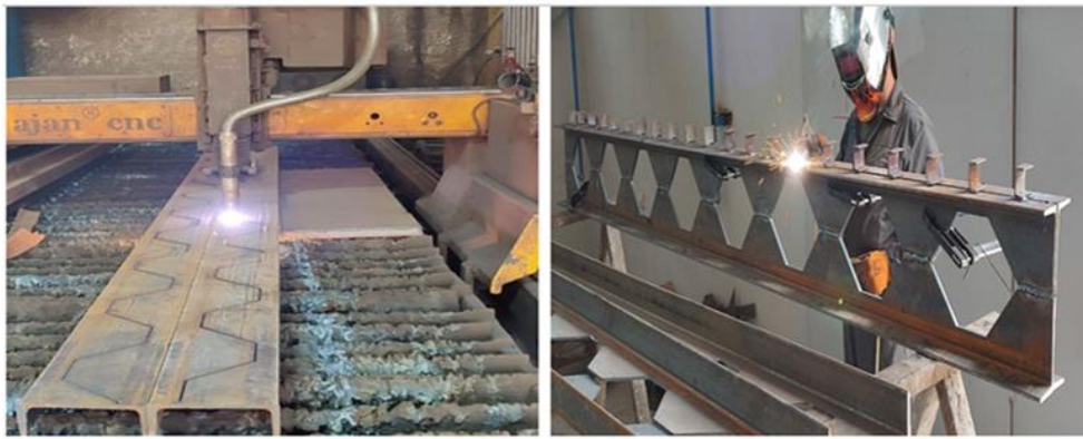
(a) Cutting by (CNC) plasma machine. (b) formation of the castellated steel beam.
