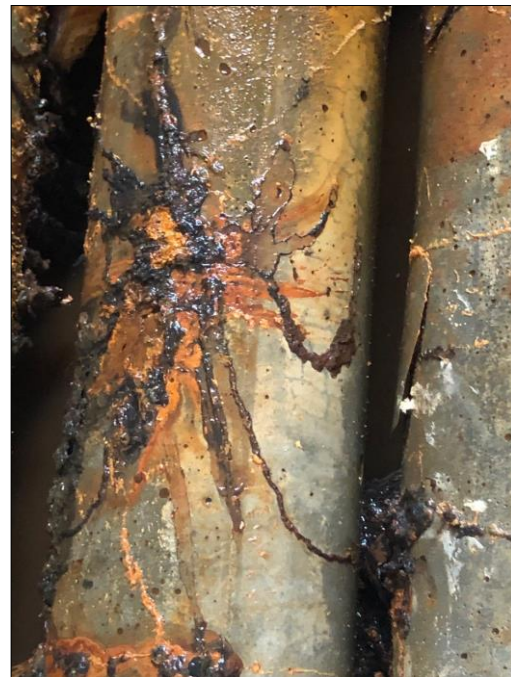
Fig. 9 10 mm Cover Cracking.
