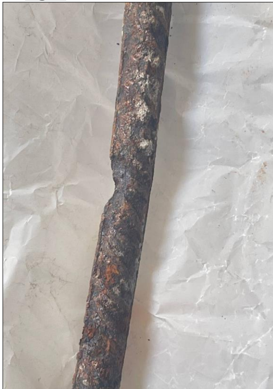
Fig.11 Corroded Steel Bar.
