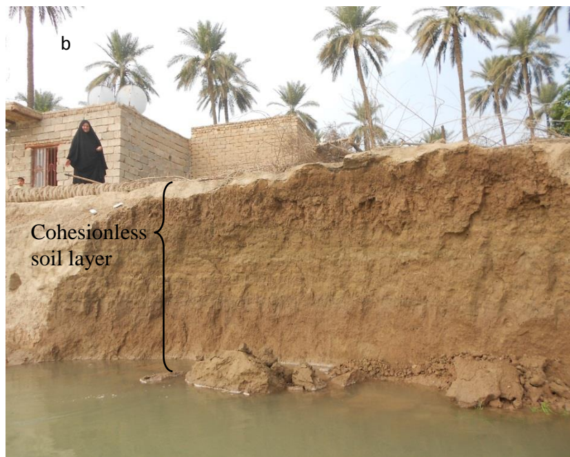
Fig. 2-b Bank erosion and their effects on settlement land put peasants' houses under tangible dangerous. The distance between the house and the new river bank is (5 Meters).
