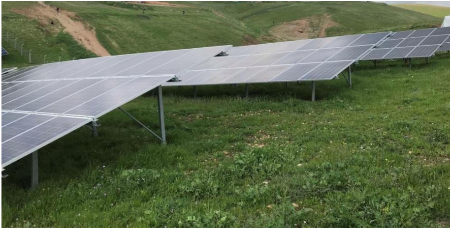
Fig. (3): A sample of the solar panel installed on the study area.
