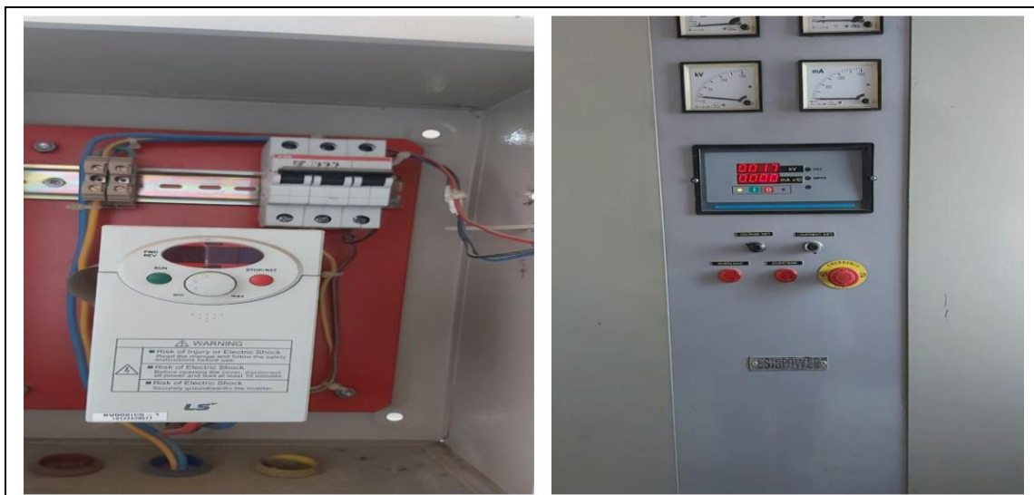
Figure 8. ESP Control Room
