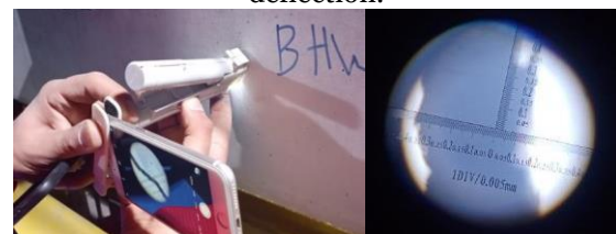
(c) Micro crack width (camera system).
