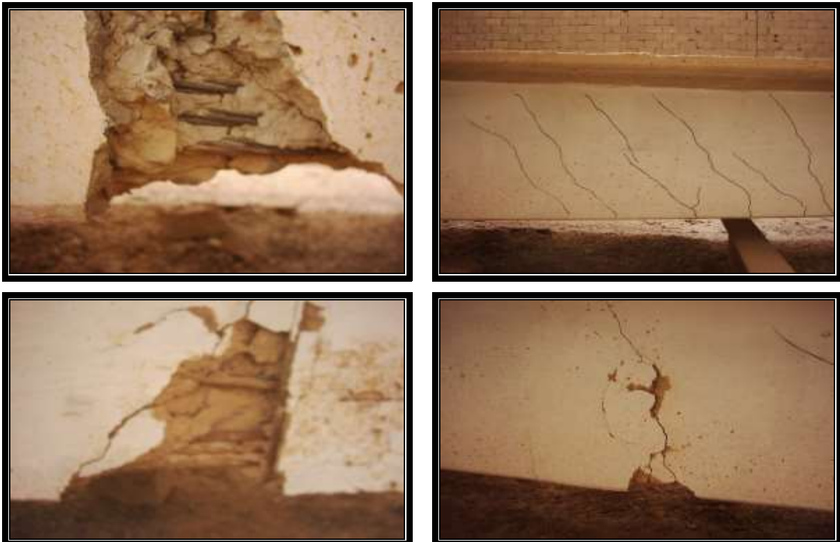
Fig. (22). Beam B3- Crack propagation on beam face side.
