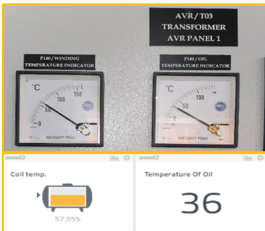
Fig. 25 Reading of the transformer panel and Cayenne dashboard
