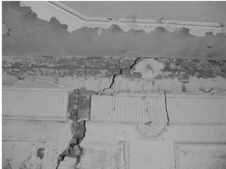
Fig. 3: Cracks in the Wall of Main Hall
