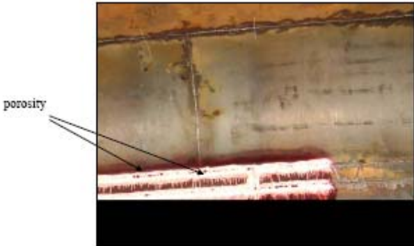
Fig ( 7 ) welding defects – porosity.
