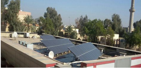
Fig. (1) 15kWp HIT Solar System Grid- tied
