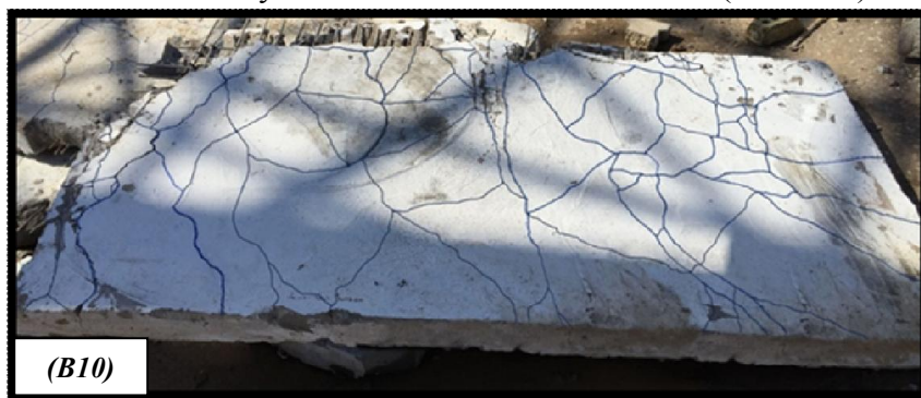
Figure (14): Crack Pattern ( D/t = 0.6 ) (B10).
