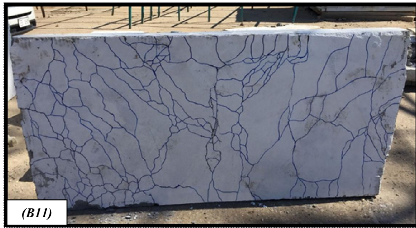
Figure (15): Crack Pattern ( D/t = 0.7 ) (B11).
