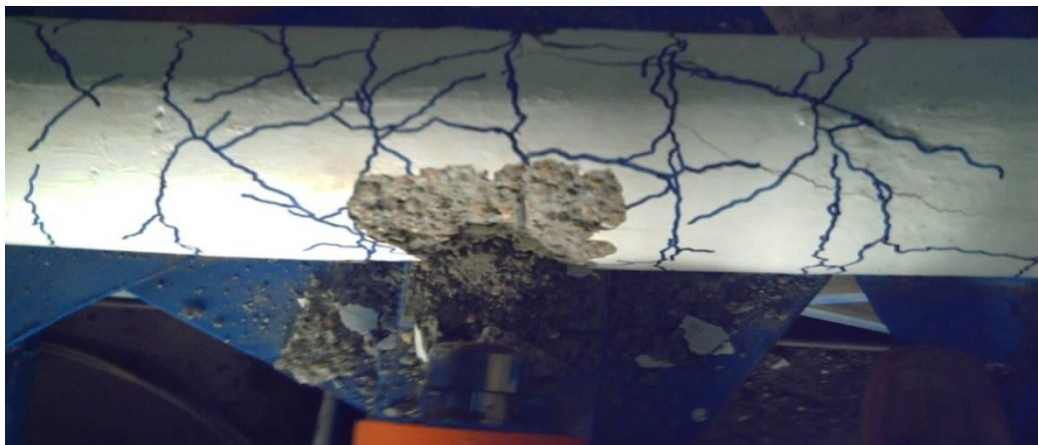
B-2 development of cracks at the upper face of column C5
