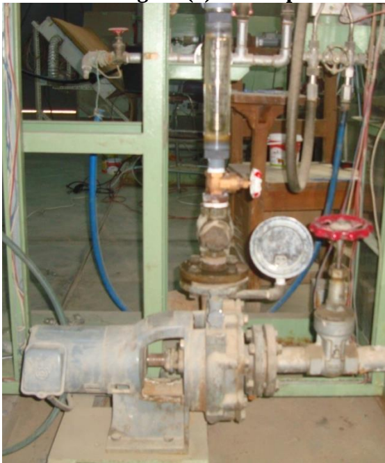
Fig (2)The pump and flow meter
