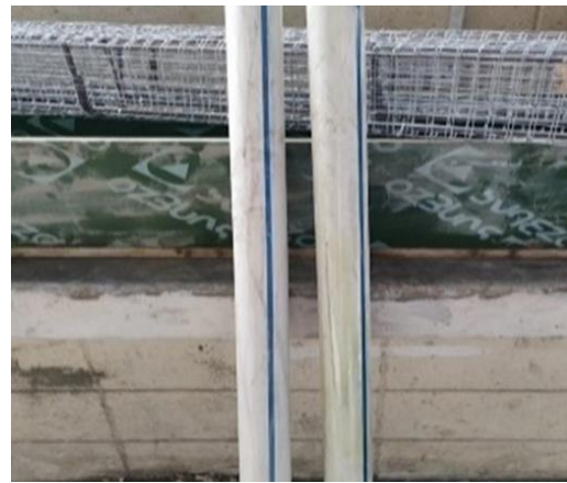
Fig. 4 Polyvinyl chloride pipe (PVC)
