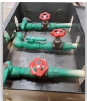
Fig. 7 The pressure control valves.
