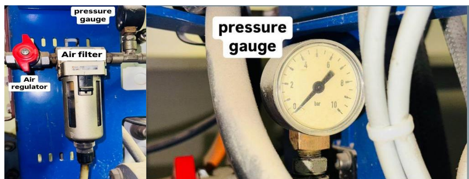
Fig. 6. Pressure gauge and air regulator.
