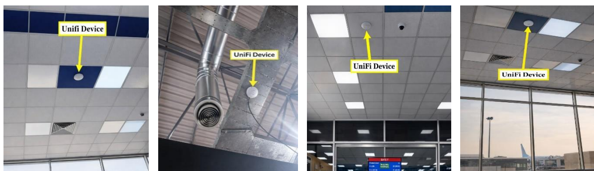
Fig. 4. The UniFi devices have been installed in real practice in the passenger terminals at various heights.
